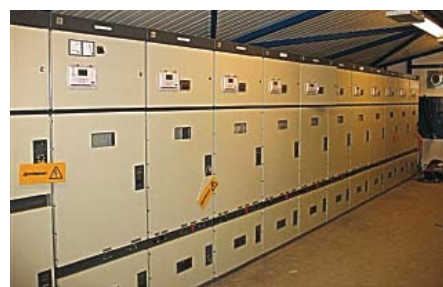
The Oulunsalo substation is equipped with 13 Vamp 255 protection relays.
